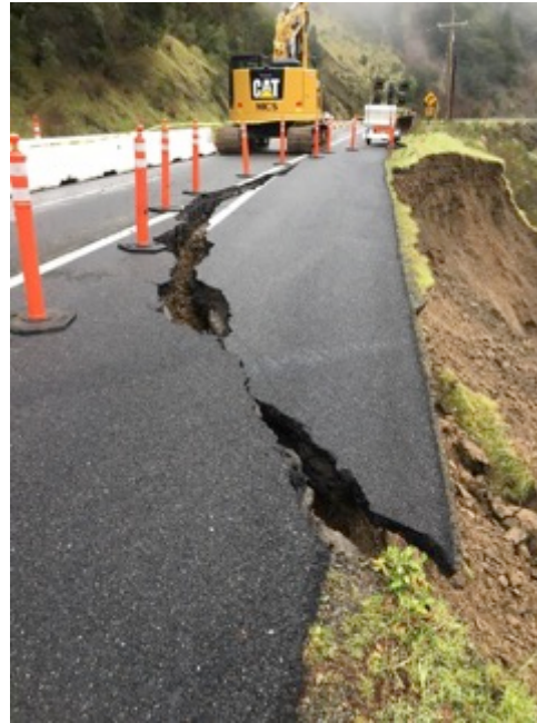
PAVEMENT CRACKING HIGHWAY 101 NORTH OF LEGGETT
