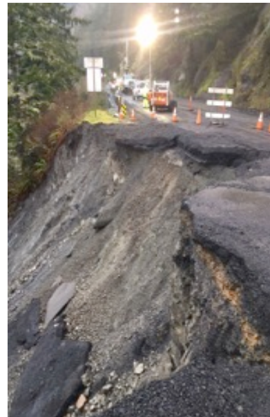
ROADWAY EROSION CAUSES DETOURS
