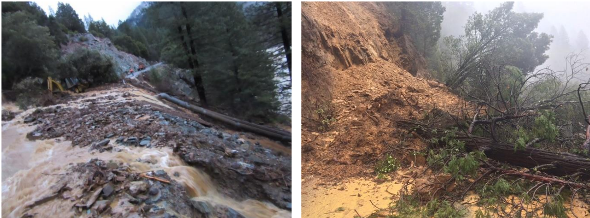
FIGURE 4: STATE ROUTE 96 STORM DAMAGE IN SISKIYOU COUNTY
