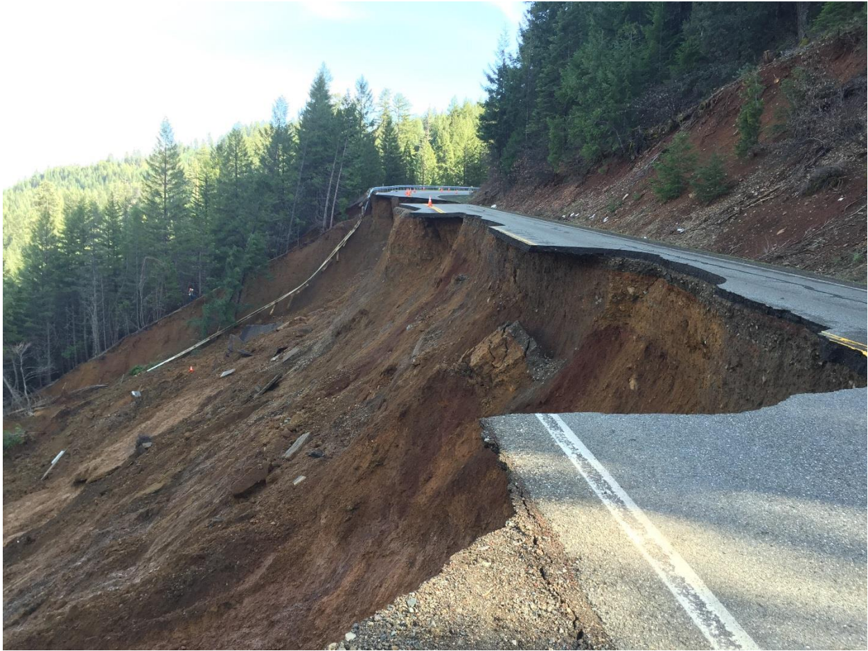
FIGURE 2: HIGHWAY 3 IN TRINITY COUNTY ROAD AND SLOPE FAILURE FROM INCREASED PRECIPITATION
