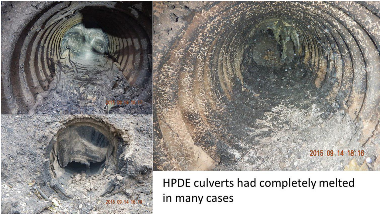
FIGURE 10-3: MELTED CULVERTS DUE TO WILDFIRES
