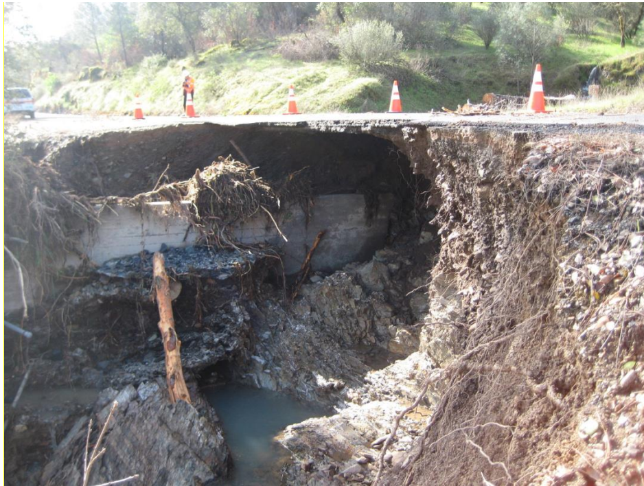
FIGURE 26: DAMAGE ON SR 49 IN TUOLUMNE COUNTY, MARCH 2018
